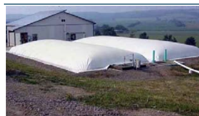
Figure 24. Anaerobic Digester, Clymer, NY
