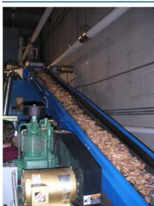
Figure 16. Wood-fired boiler, Hanover, NH
